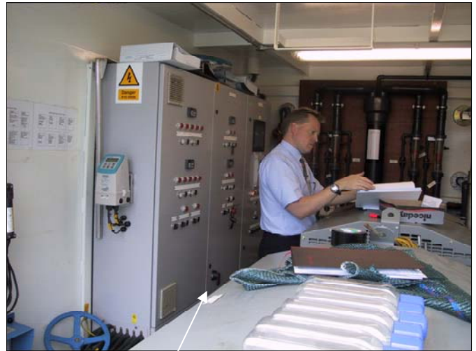
The main isolator
